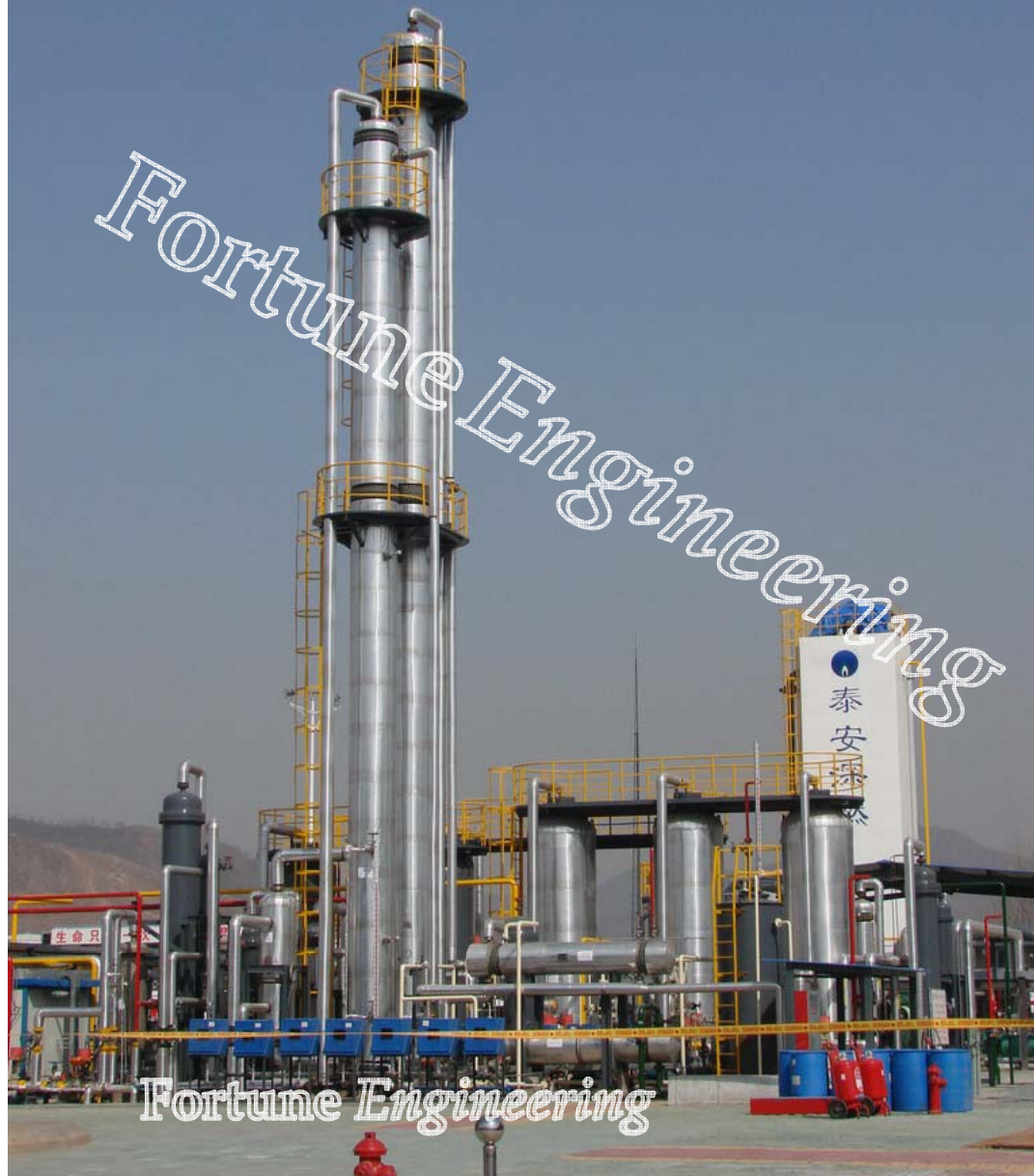
Full Layout View of The Plant - 3
