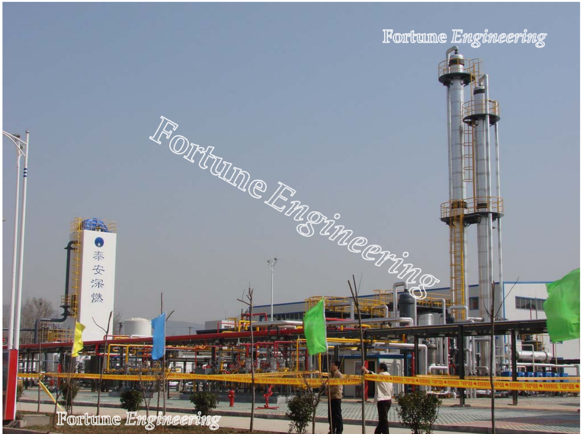
Full Layout View of The Plant - 2
